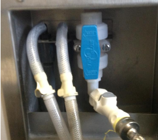
1" air gap maintained
